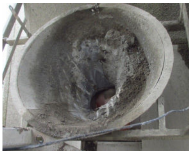
Example of build-up in steel chute
