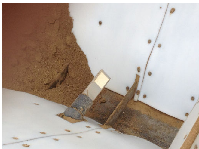
Hydronix probes were installed in the sand bins
