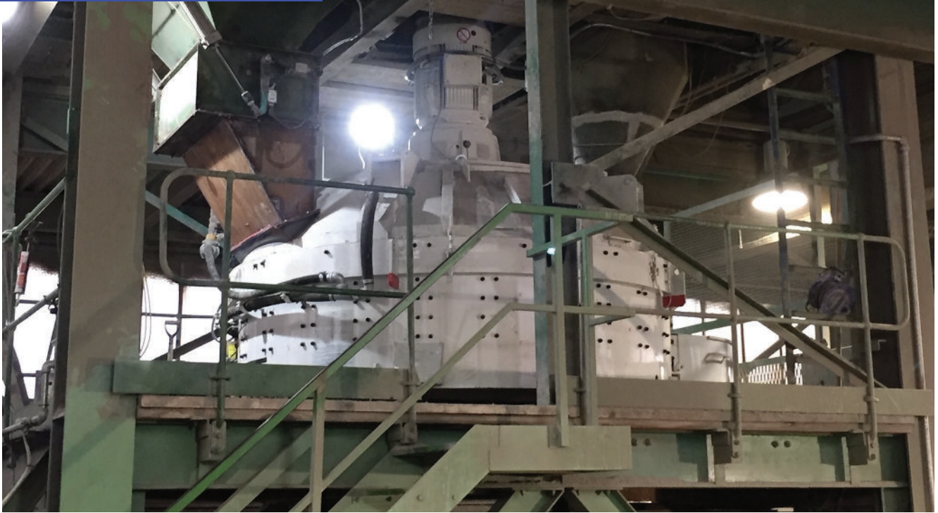
One of Besblock's new TEKA planetary mixers, supplied and installed by ConSpare
