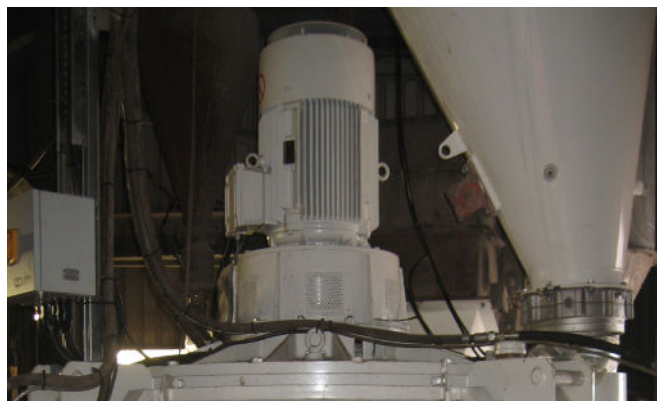
82kW drive system reduced to 45kW with Teka TPZ1500
