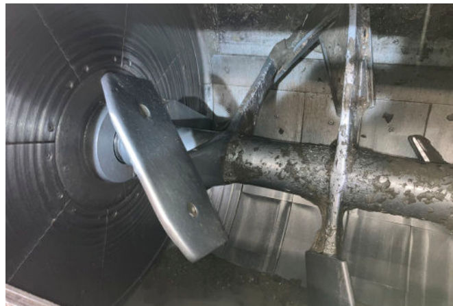
Single shaft mixer following automated cleaning cycle
