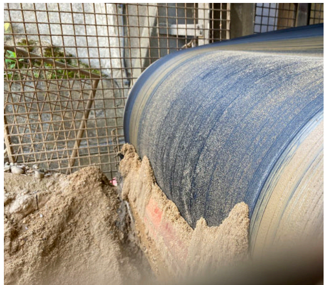
Ineffective belt scraper covered in carryback
