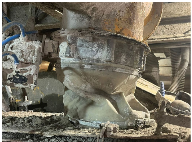
Jubilee clipped connector on cement inlet above mixer
