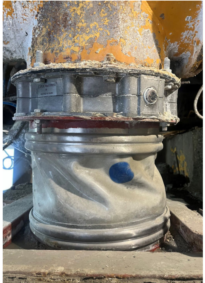
BFM® fitting installed on cement inlet above mixer
