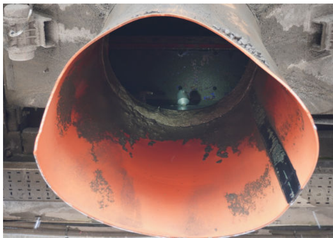
Autonomous chute cleaner eliminates blockages
