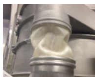
Installation gap too small
