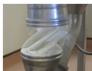
Installation gap too large
